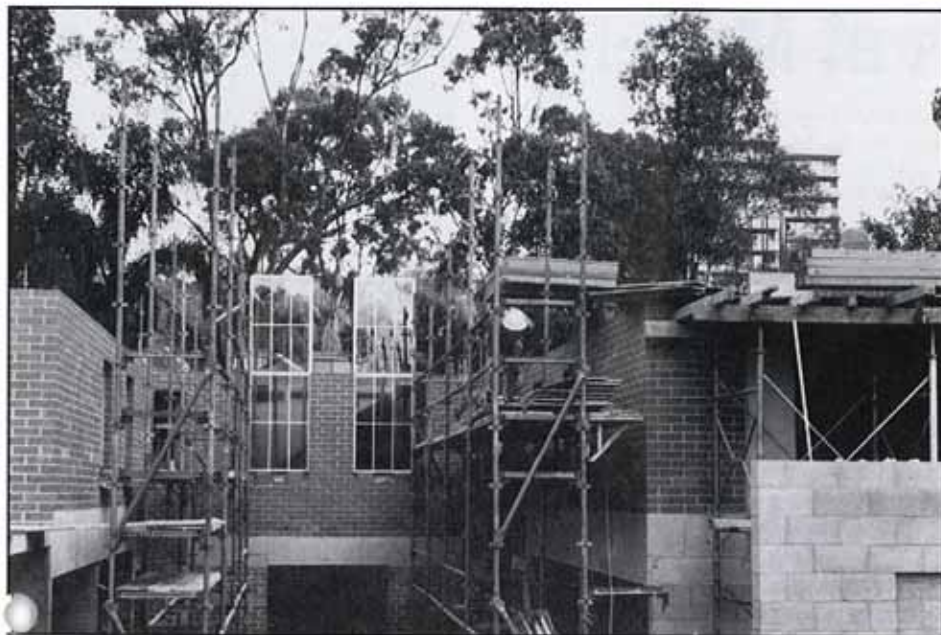
Work is progressing well on these top quality units in Jerdanefield St, St Lucia.
